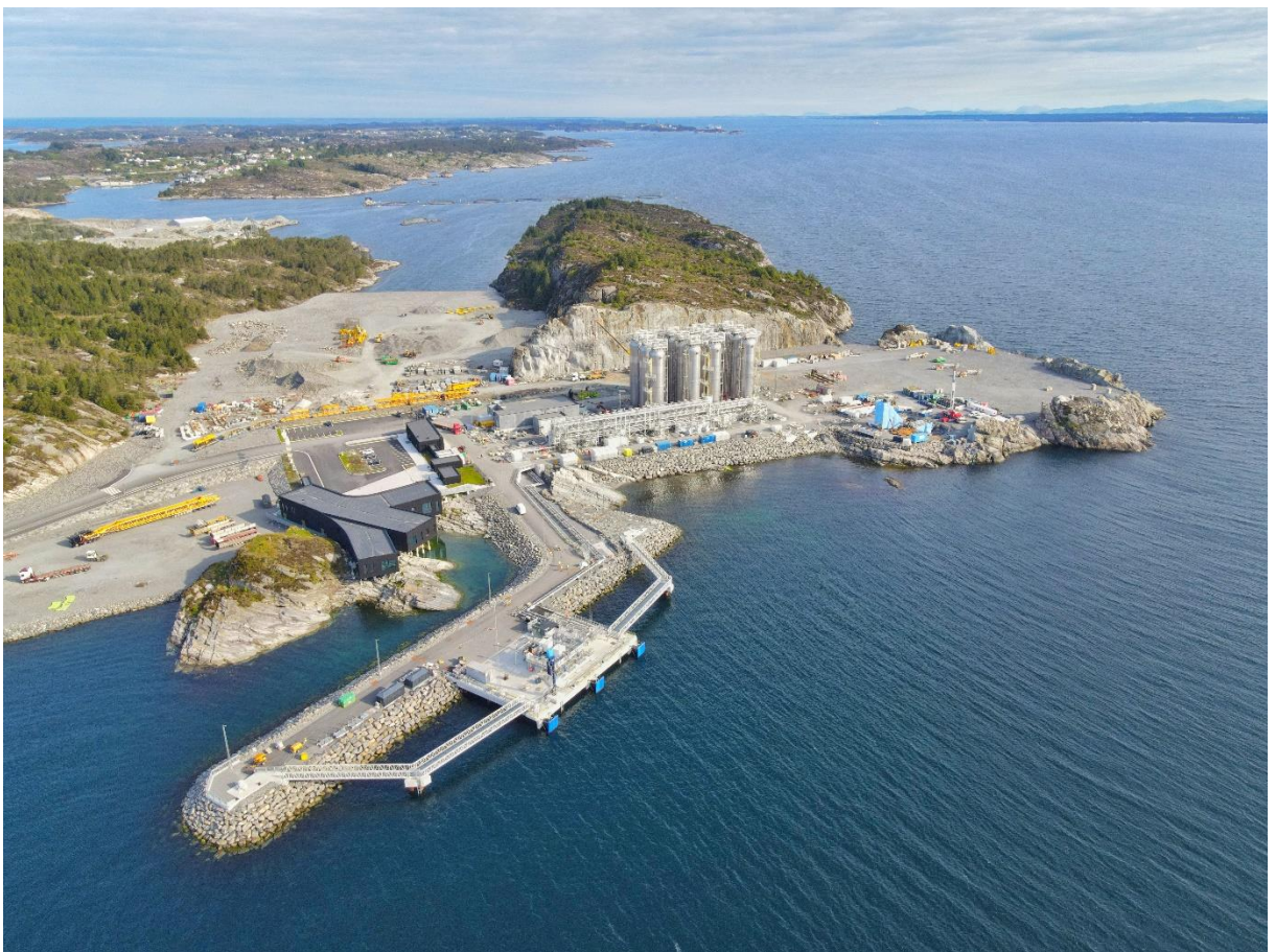
Northern Lights' CO 2 receiving terminal in Øygarden.
