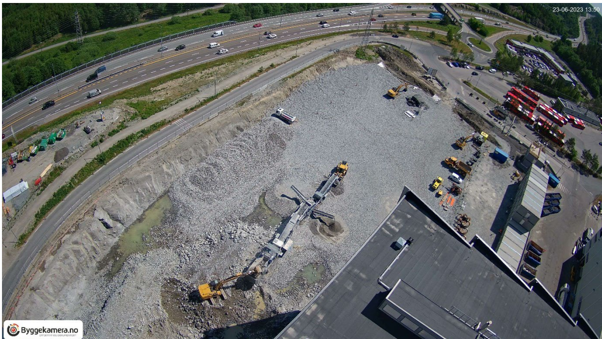
Ground works on site at Hafslund Celsio's waste incineration plant in Oslo.
