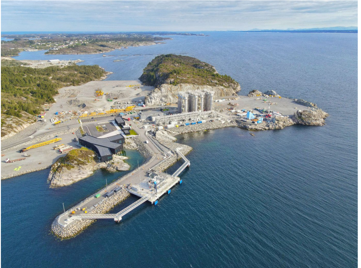
Northern Lights' CO 2 receiving terminal in Øygarden.
