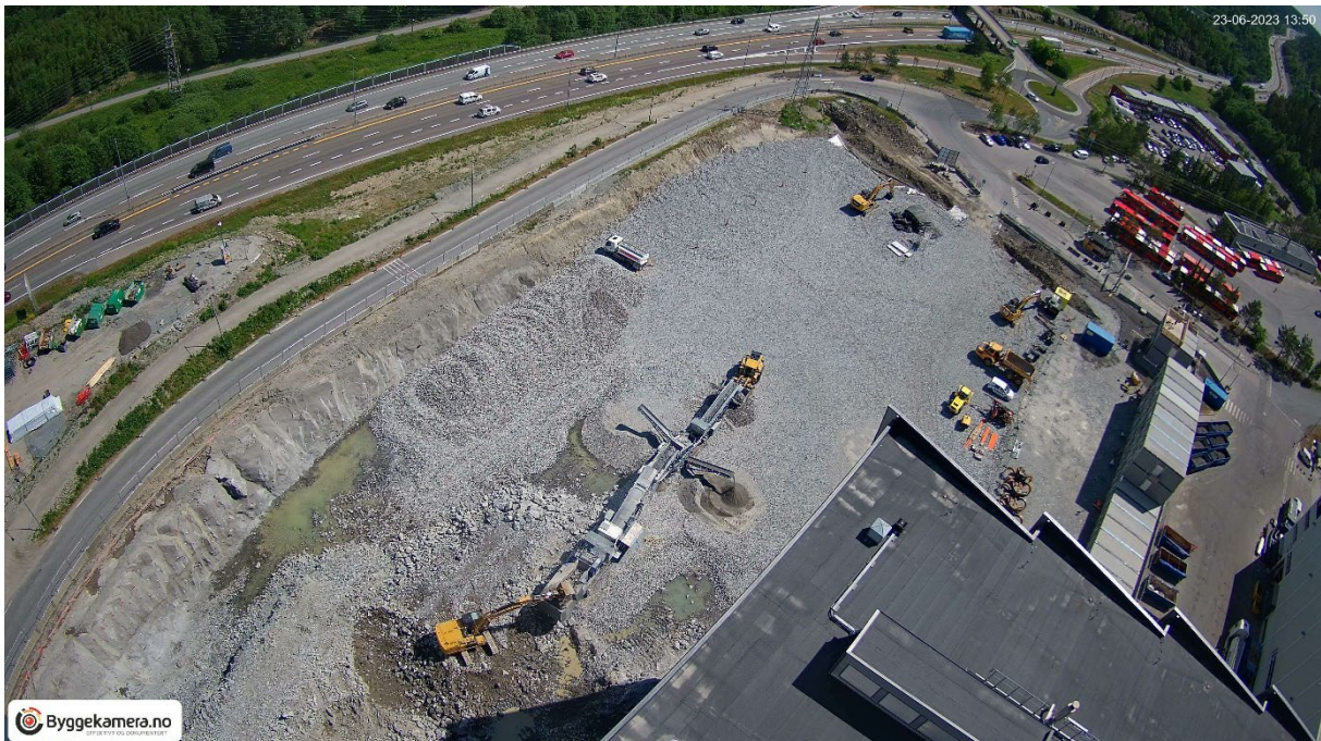
Ground works on site at Hafslund Oslo Celsio's waste incineration plant in Oslo.
