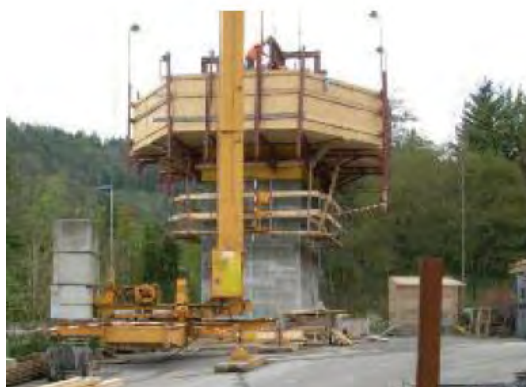
Figure 6 Picture of slip forming mock-up with actual design and dimensions of concrete absorber with liner
