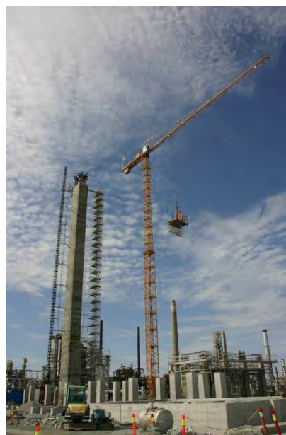
Figure 2 Picture of construction of the amine unit with finalized slip formed absorber
