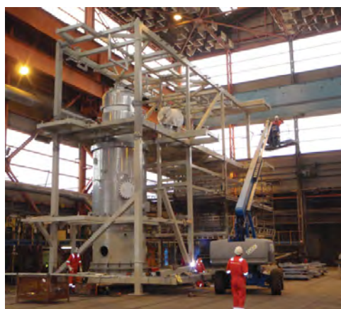
Figure 3 Picture of construction of one reboiler on a pre-assembled unit at the Aker Stord yard
