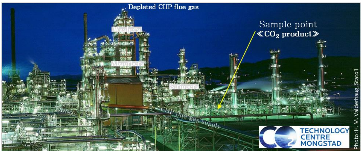
Fig. 1. Technology Centre Mongstad (TCM), Norway [Photo © Equinor] DA amine plant with CHP flue gas inlet from the front, and the high absorber tower in the middle. “Captured” CO 2 product outlet and sample point towards the right.
