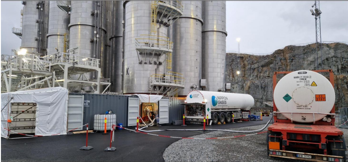
Unloading CO 2 from Trucks to the facility
