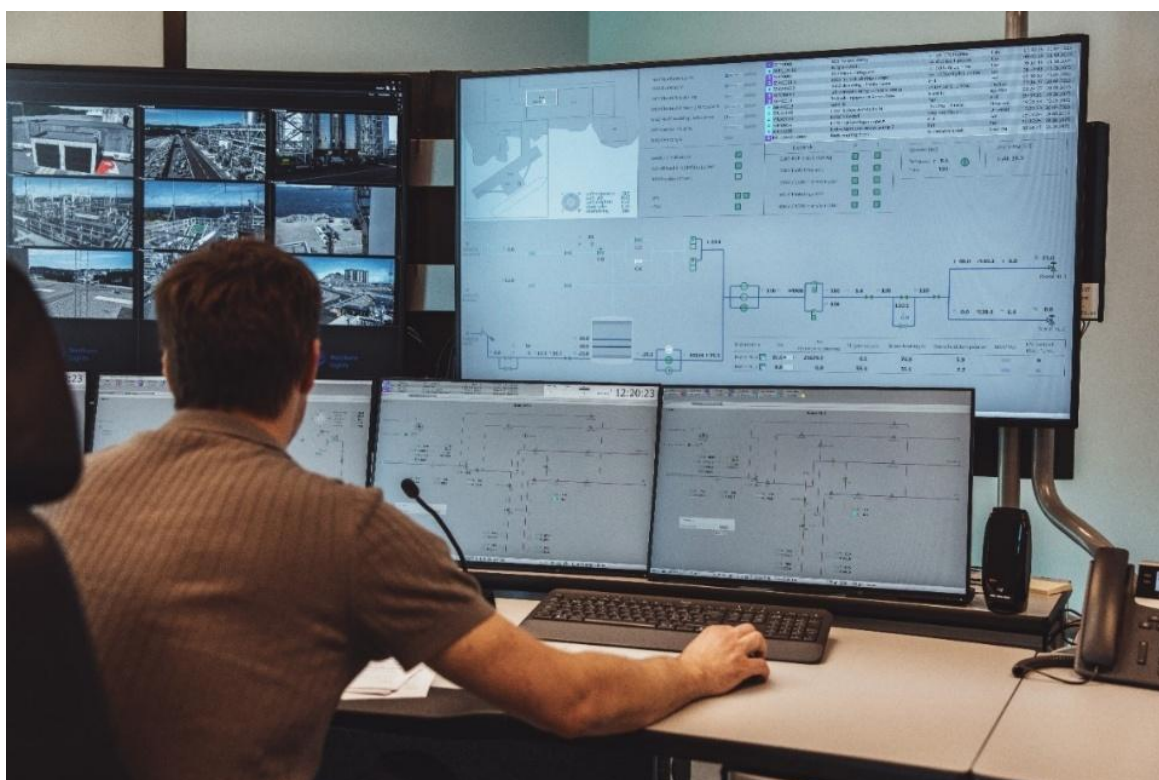
Monitoring from the control room at the Øygarden CO 2 receiving facility to monitor that the CO 2 has been injected into the reservoir.
