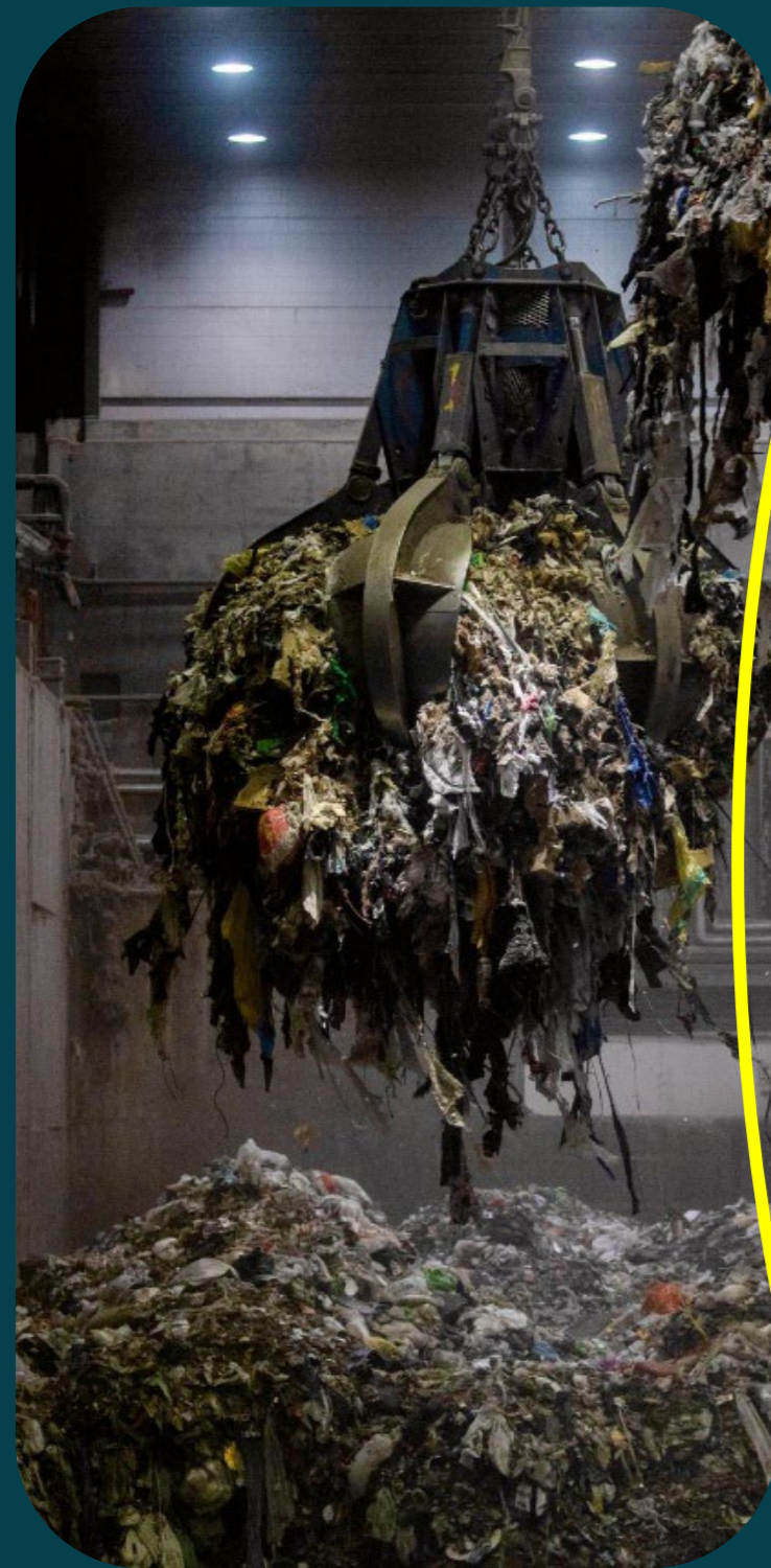
Norway's largest waste incineration plant (350 000 t/Y)
